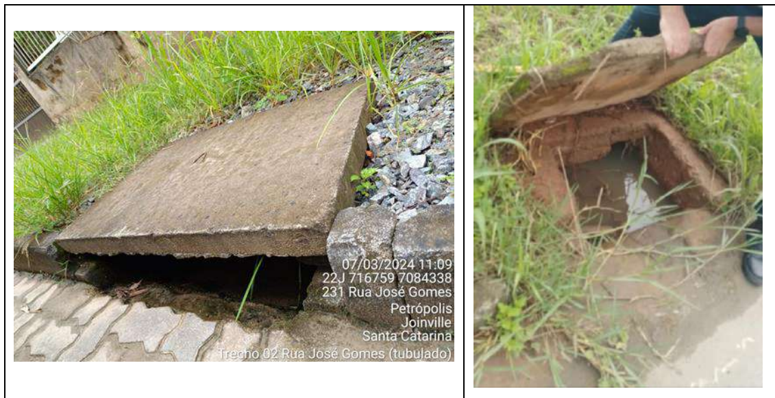
Figura 16: Bueiros na rua lateral José Gomes (716759.60 m E, 7084266.52 m S) e na principal Jacinto Machado (716983.27 m E, 7084346.51 m S).
